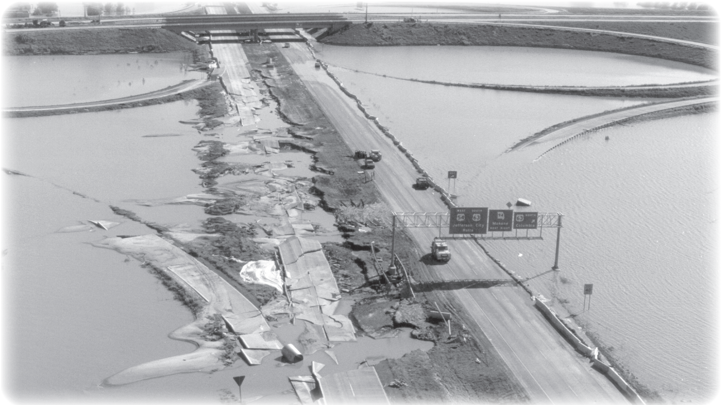
Flood waters destroyed roadways across the state in 1993. Pictured is MO Highway 54 in Jefferson City.
