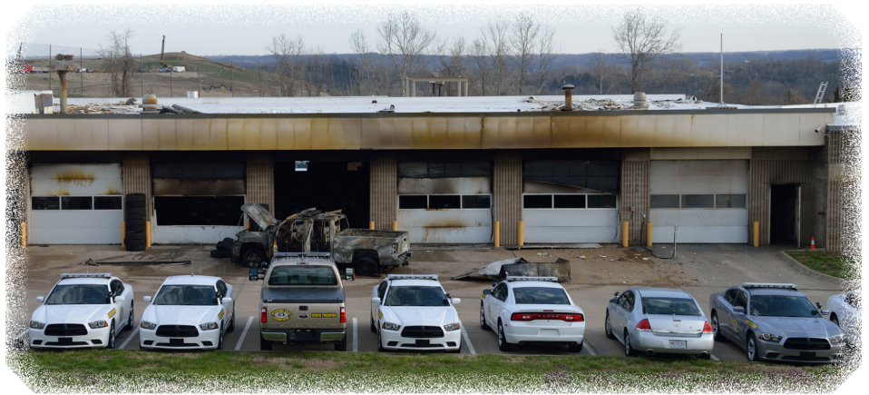
A fire destroyed the GHQ Garage on April 8, 2014, including 10 work bays, the car wash, and the warehouse and vehicle detail area. The Radio Shop (east end of the building; not pictured), which sustained smoke damage, was operational within a few days.
