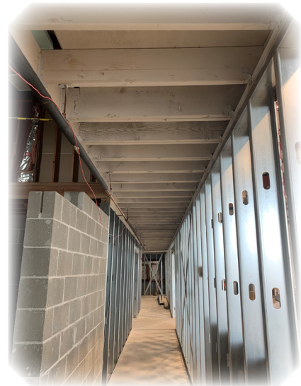
This photo shows the steel framing, safe room location, and exposed ceiling on July 16, 2020.
